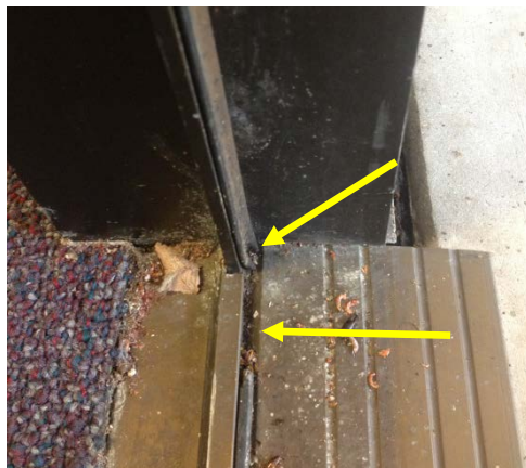
Fig 2. Worn and improperly installed weather stripping. Photos: Mike Bentley
