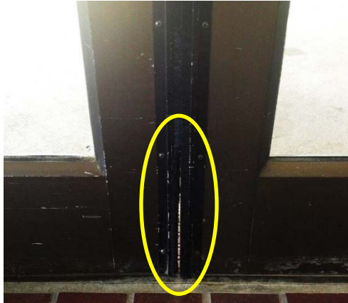
Fig 1. Air gap in doors.
