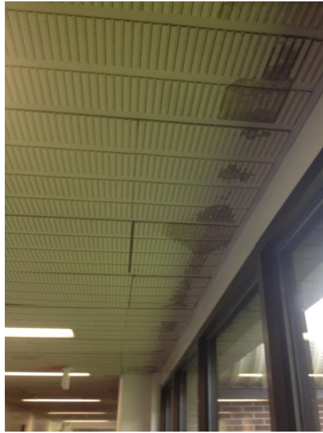
Fig 1. Evidence of moisture intrusion visible through ceiling tiles. Photo: Mike Bentley
