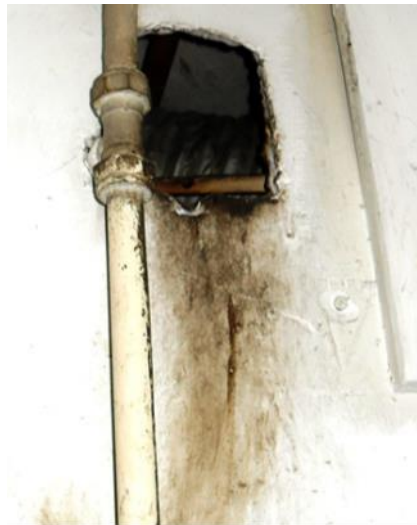
Fig 2. Rub marks made from repeated entry into a structure by rodents. Photo credit: www.Rentokil.co.uk
