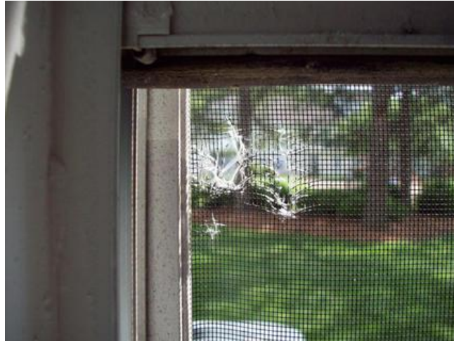
Fig 2. Damaged screen that can create an easy access point for flying pests to enter a structure. Photo credit: Kudzu.com.
