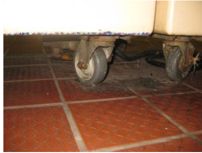
Fig 2. Floor under serving line after end-of-school "deep clean." Is that a tater tot? Think there is enough in the wheels to sustain German cockroaches?
