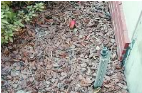
Fig. 2. Mulch that is too thick and obscures an inspection space will result in what is termed a “conductive condition” in the pest control industry. The irrigation head depicted here is in violation of the current building code. The Florida building code requires that irrigation be installed 1 foot or more away from a building sidewall. Irrigation heads that “water walls” is also considered a conducive condition.
