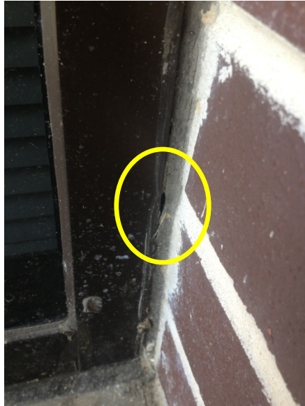
Fig 3. Old caulking. Photos: Mike Bentley
