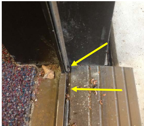
Fig 2. Worn and improperly installed weather stripping. Photos: Mike Bentley
