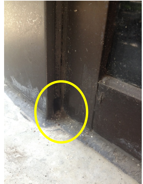
Fig 4. Gap in caulking bead.
