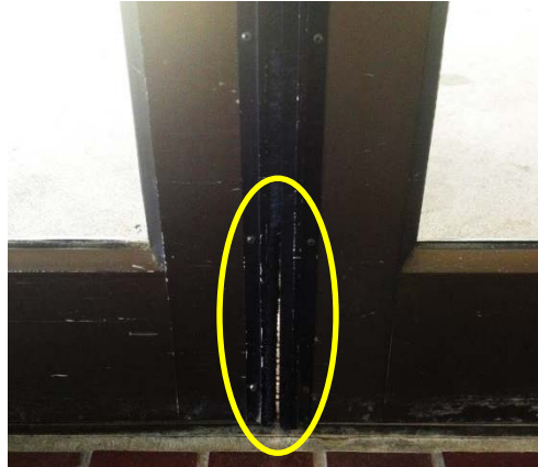
Fig 1. Air gap in doors.
